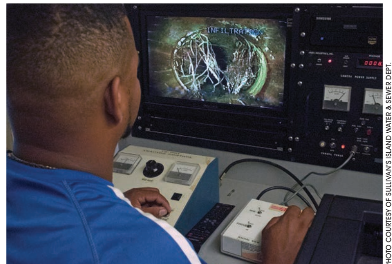
Darrell Noisette pauses to view an infiltration source while inspecting a sewer main on Sullivan's Island.
