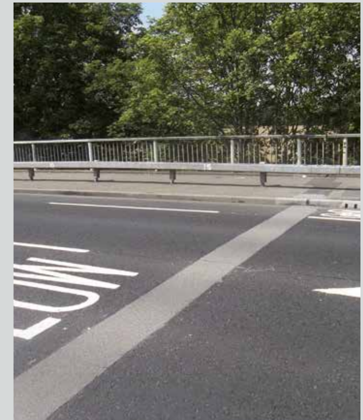
FEBA joint extends across the full length of the carriageway and into the verges.
