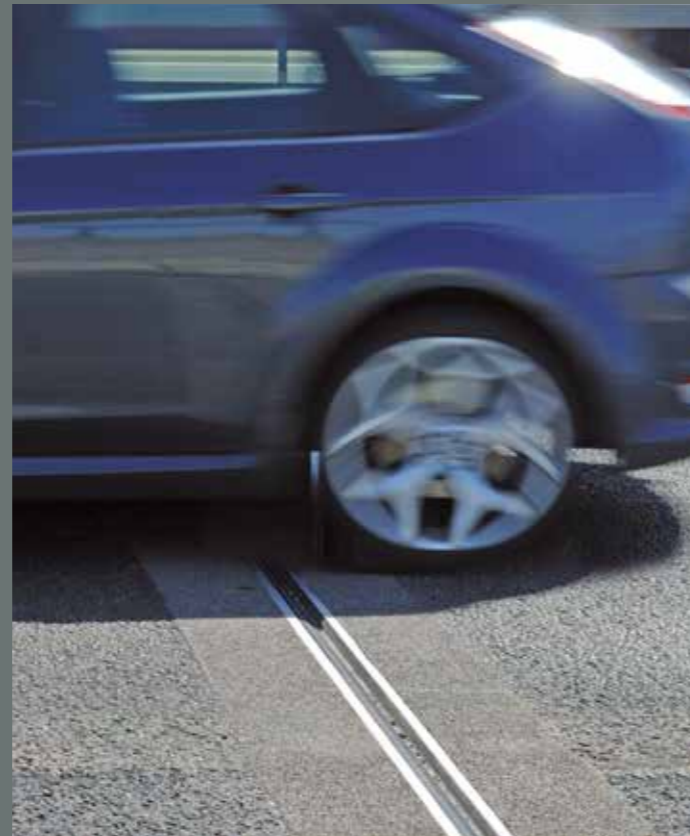
A close up of the BEJ expansion joint system not normally seen by the travelling public.
